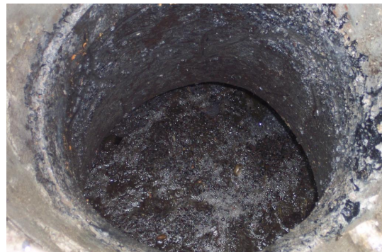
Photograph 5. Inside view of digester
