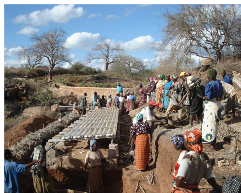
Photograph 2. solar disinfection system installation almost complete
