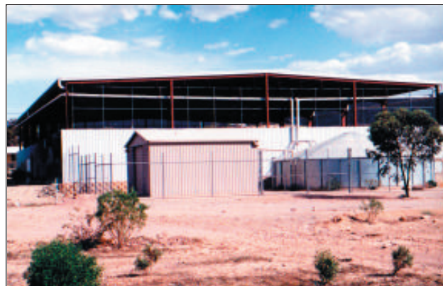
Photograph 1. Rainwater collection, storage tank and ultraviolet light treatment plant at the Nepabunna basketball stadium
