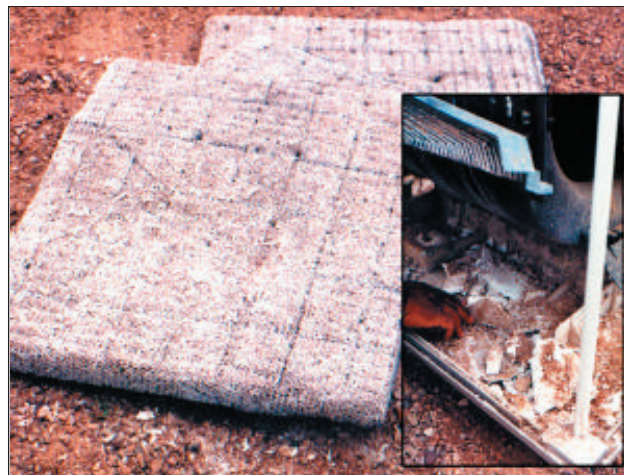
Photograph 2. Filters from water-based air coolers clogged up with salts (inset: salts accumulating at the base of a cooler)
