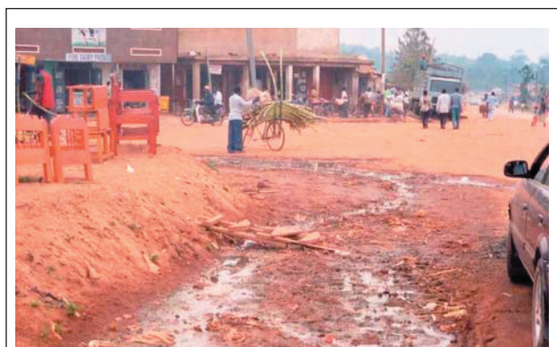
Photograph 1. Surface runoff needs managing
