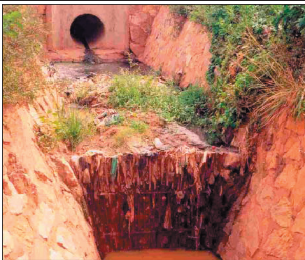
Photograph 4. A blocked drain
