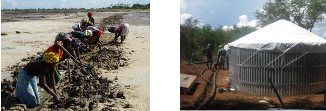
Figure 2. Community engagement during construction phase (left) by digging trenches for more than 6 km for the pipelines. Storage tanks of a type also used in emergency response, but with long lasting quality were installed to enable storage capacity of at least 40 cubic meters (right).
