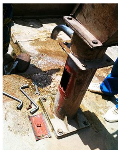
Photograph 2. An India Mark II handpump modified for installation of level loggers
