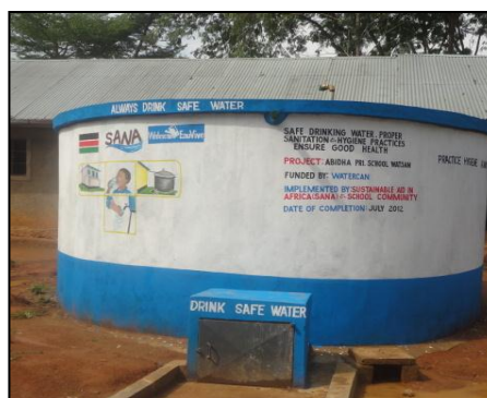
Photograph 3. Rain Water Harvesting System at Abidha PS
