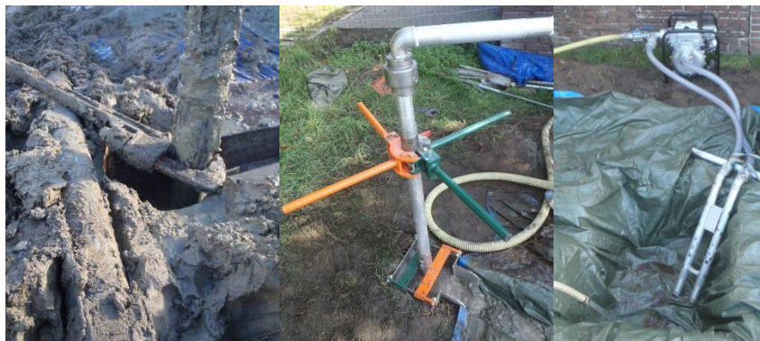
Photograph 4. a) Way of fixating drill string in developmental context. b) Improved fixation. c) Inlet and outlet in the mud pit. 3
