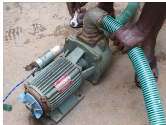
Photograph 2. Centrifugal pump external to a pit
