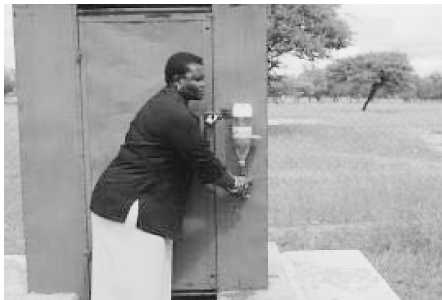
Photograph 4. CSIR Hand Washing Dispenser installed outside the sanitation facility (CSIR, 2004)
