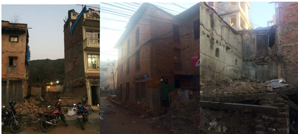
Figure 3 Images of Banepa's damaged building stock (authors' pictures)
