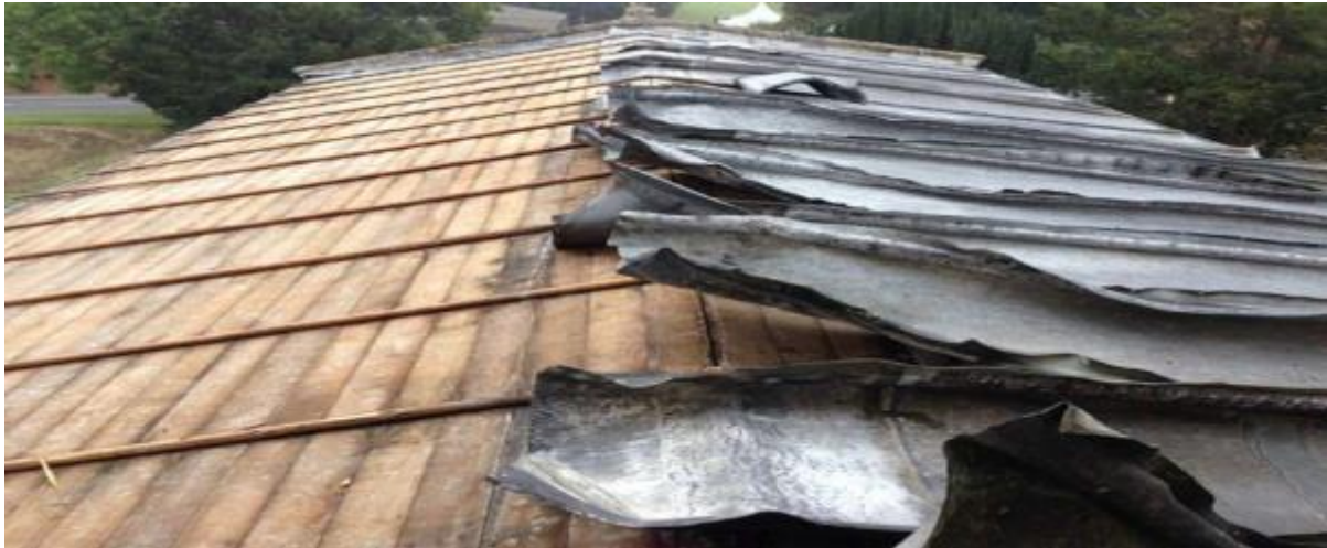
Figure 1 – A church roof which has been a victim of lead theft[7]
