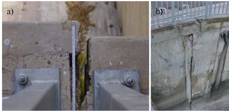
Fig. 3. a) Relative displacement in block 13-14 (downstream face) and b) joint 13 in the upstream face.
