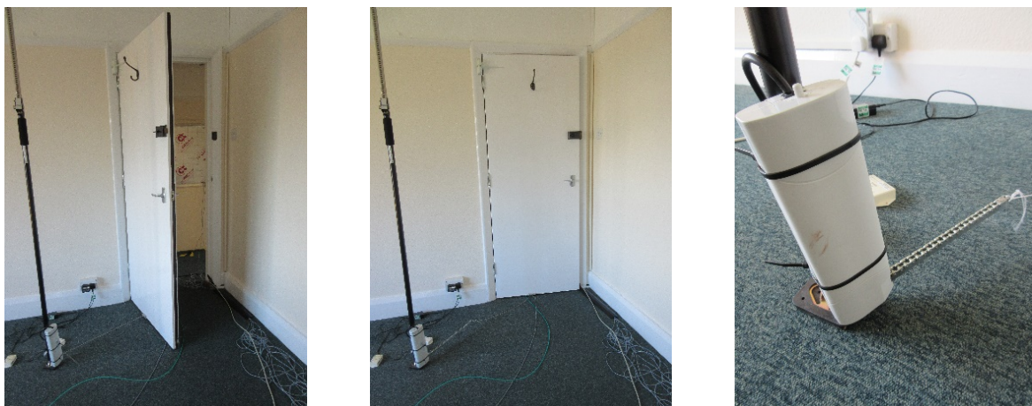
Figure 12 - Internal doors controlled by a chain actuator
