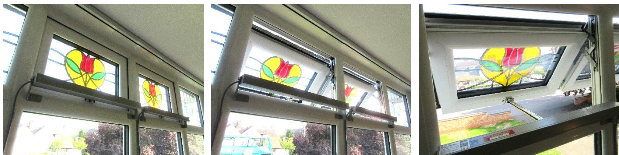
Figure 9 - Windows controlled by chain actuators
