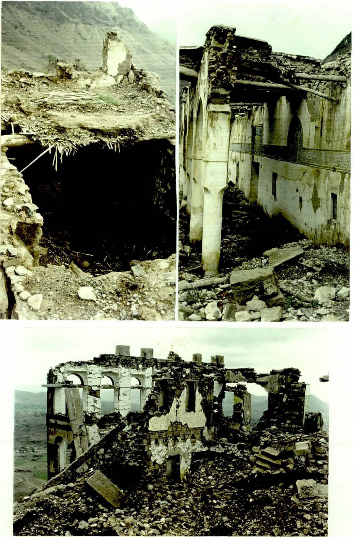
Figure 4.4: Some of the buildings damaged during the 1982 earthquake Source: Field Surveys, 1994
