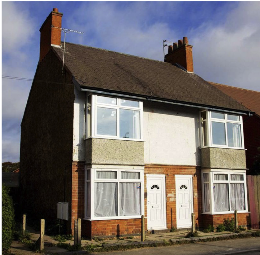
Fig. 1. The S-SE facade of the pair of Test Houses. Internal wall insulation was installed in the left house.
