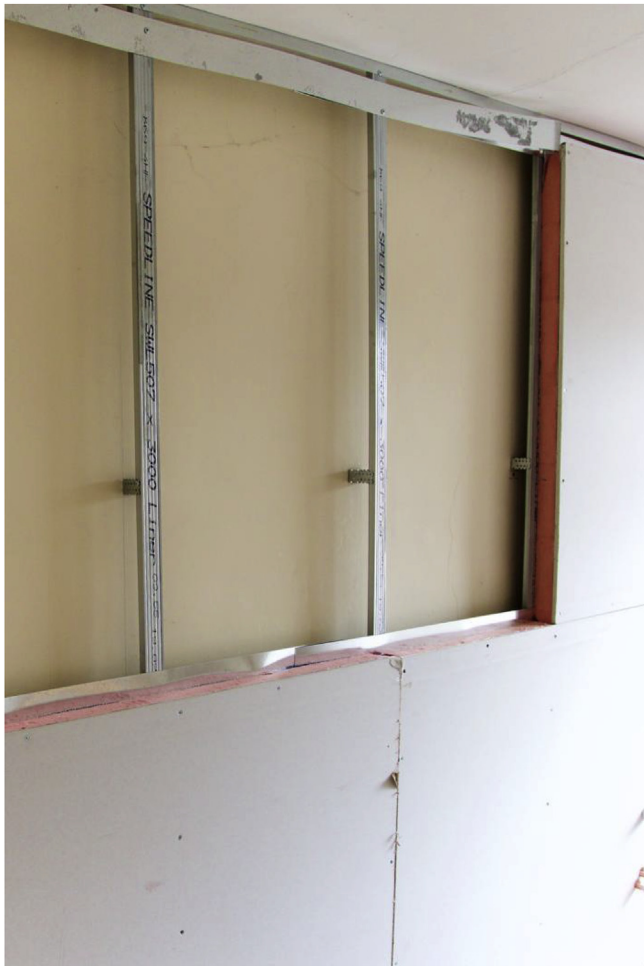
Fig. 4. The IWI system installed in the left house showing original plaster wall, air gap, steel framing and insulation panels. All joints between panels were sealed before testing.
