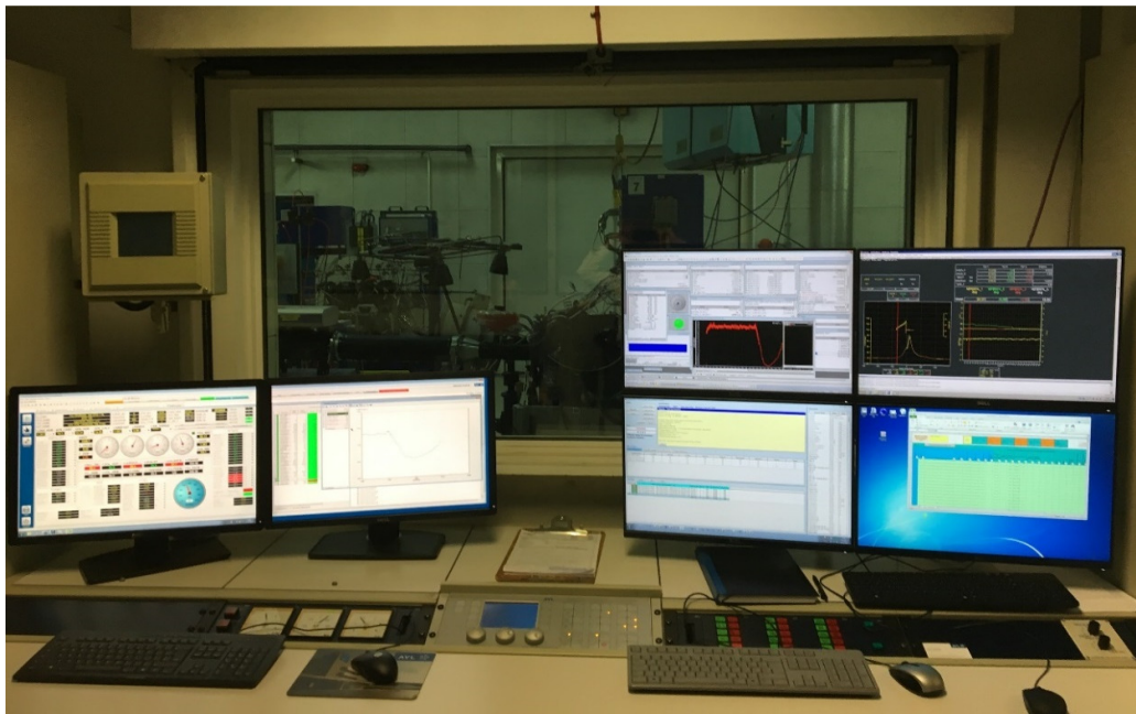
Figure 9.2: Engine test cell control panel
