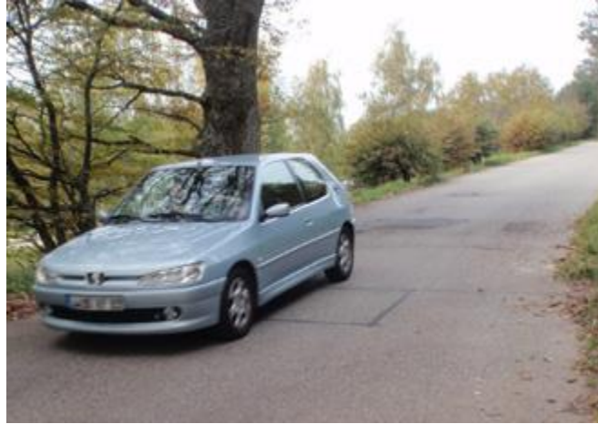
Figure 3.8 Inductive loop installed in the road ( Source: Eco Counter, Inc. )
