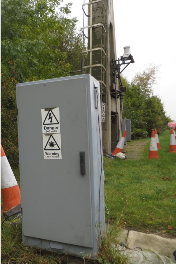
Figure C7 A Clearview Intelligence cabinet on the M1-A1 Link Road
