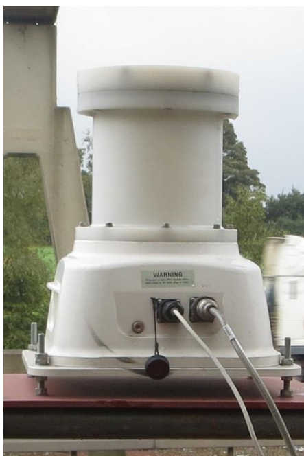
Figure C6 Ethernet (left) and power connection (right) of the radar sensor on the M1-A1 Link Road
