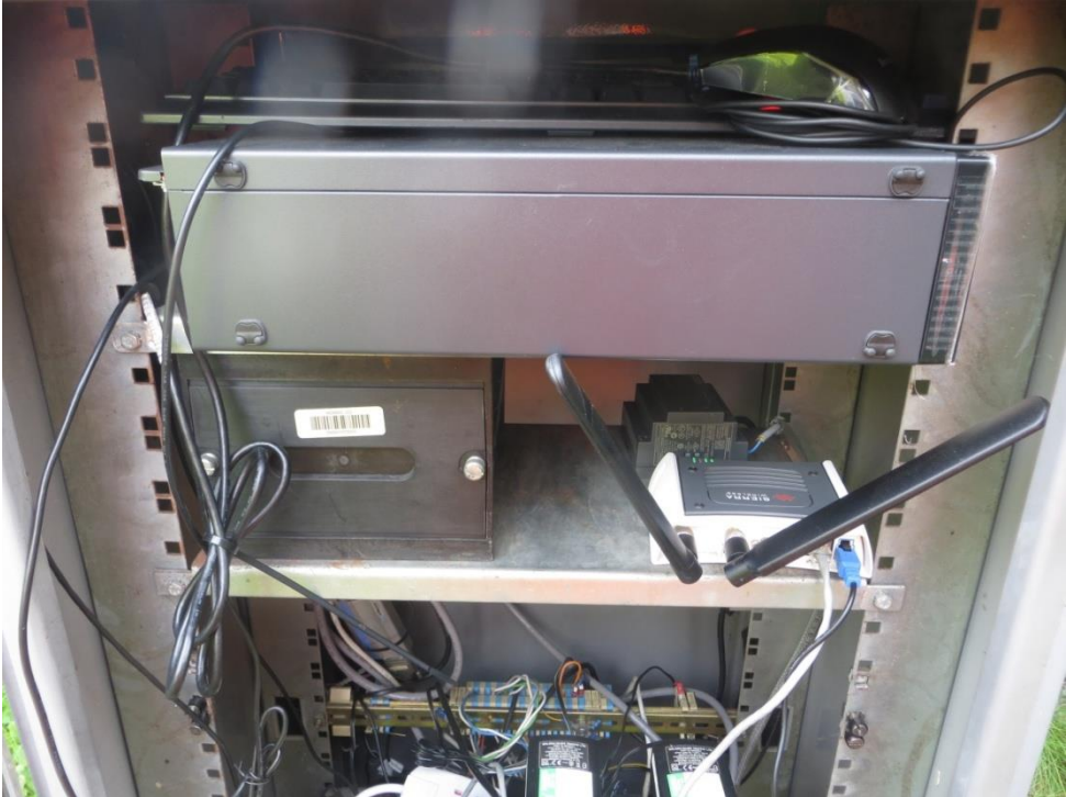
Figure C10 Server on-site (top) and router connection (bottom right) installed on the M1-A1 Link Road
