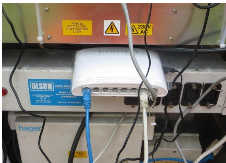
Figure C9 Ethernet switch of the radar system installed on the M1-A1 Link Road
