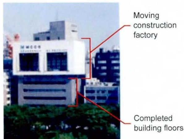
Fig. 2.14 MCCS System by Maeda Corp. during of the Sekai Bunka Sha Building in Tokyo, Japan (Maeda, 1998)
