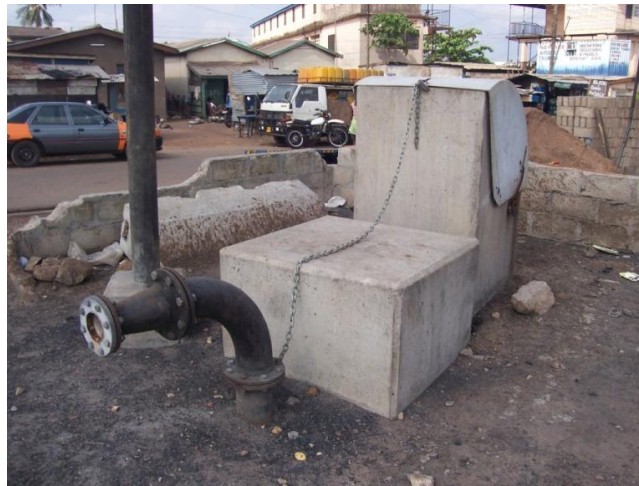
Figure 2 – An Underground Holding Tank (Photo : Niall Boot)
