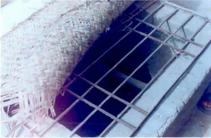
Borehole well in a Gulzar-e-Hijri location
