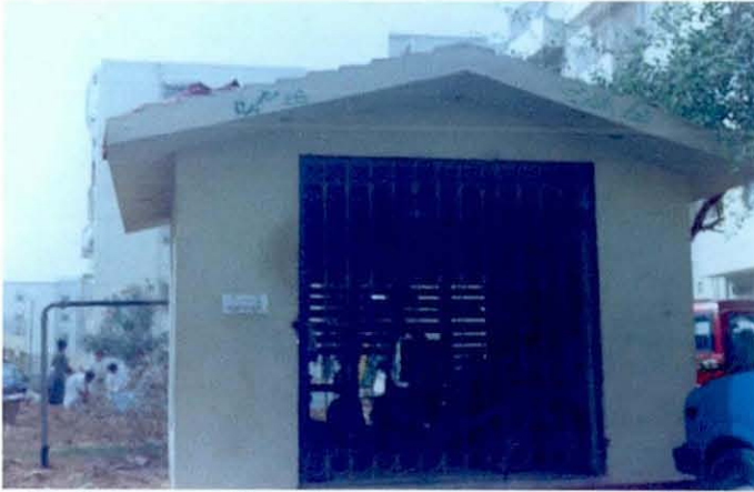
Suction pump fixed in an apartment – an enclosure constructed to protect its visibility from outsiders
