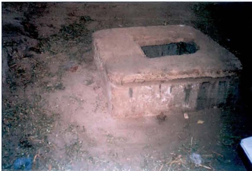
Water valve where the cover is not present
