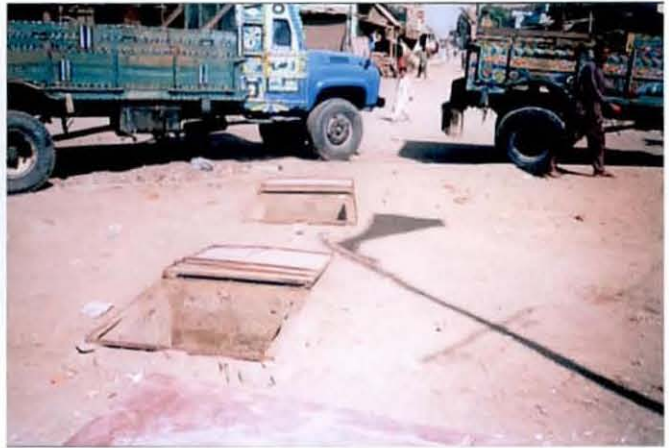
Water valves being destroyed due to the movement of trunks
