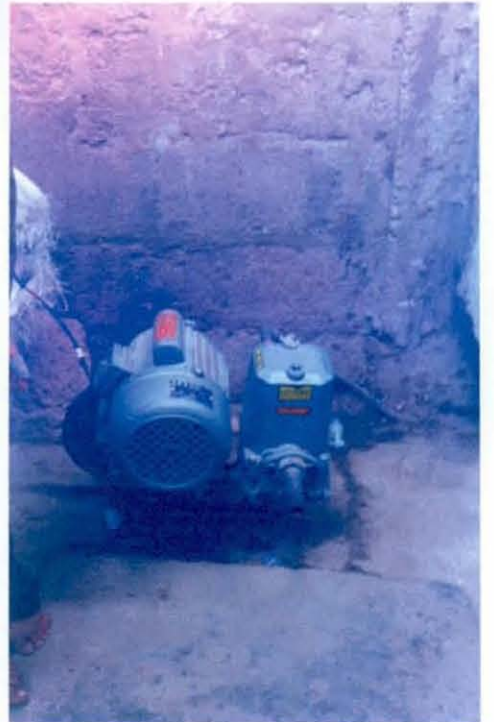
A Suction pump in a squatter settlement
