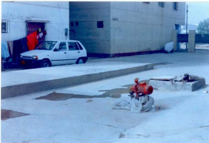
A view of a tank and suction pump
