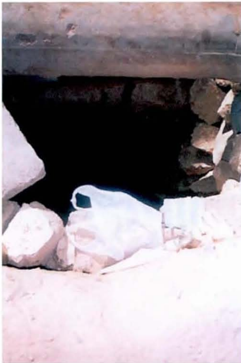
Manhole on a sewerage line
