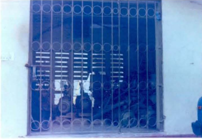
Suction pump in a high income apartment block
