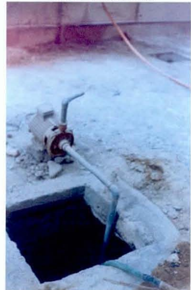
Suction pump in a new apartment
