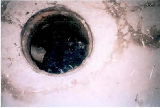
Manhole from where water line is also passing
