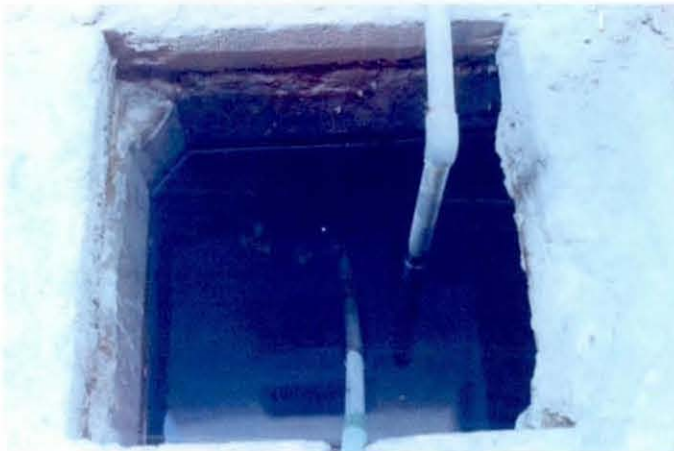
Water being transported from an underground tank to overhead tank
