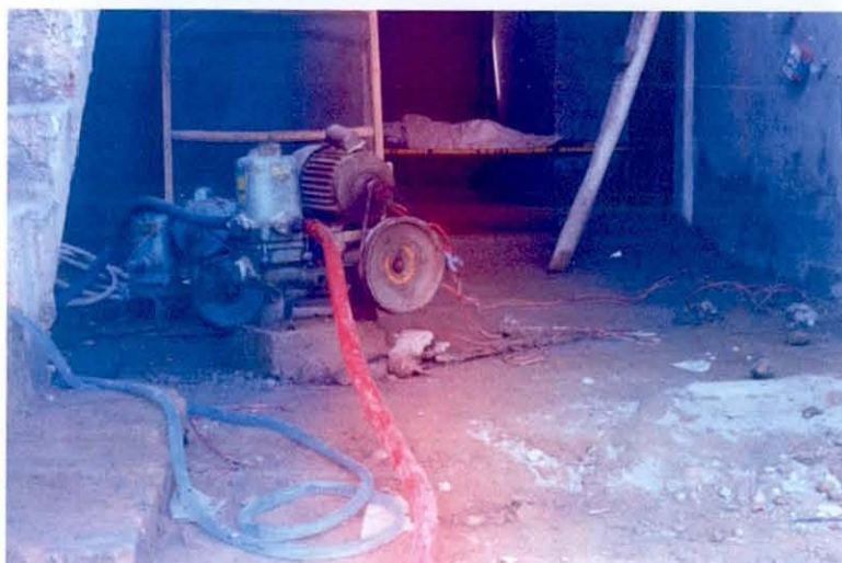
Suction pump in a squatter
