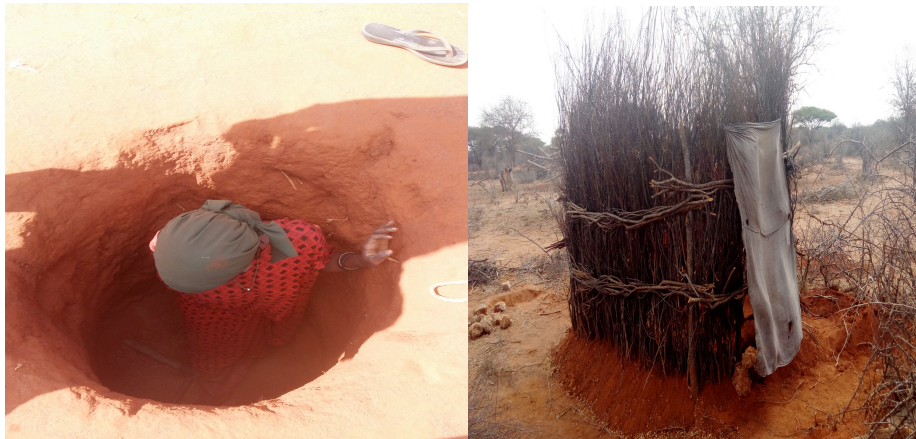
Photograph 1. A woman digs her own pit latrine (left) and the complete latrine (right)
