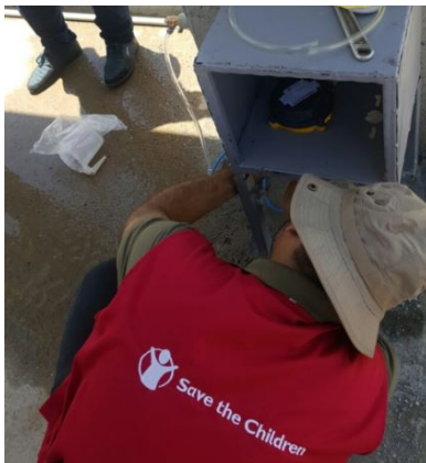
Photograph 2. A Chloroclam device being installed in Laylan II by the WASH team in Iraq
