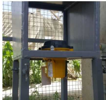
Photograph 2. A Chloroclam device installed on a pipe close to the outlet of the water source in Laylan II
