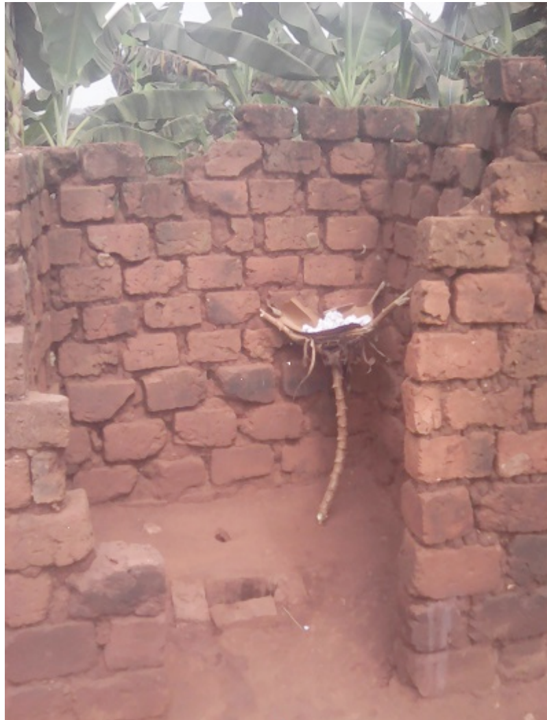
Figure 1. A causally constructed latrine, lacks universal designed components not disability friendly
