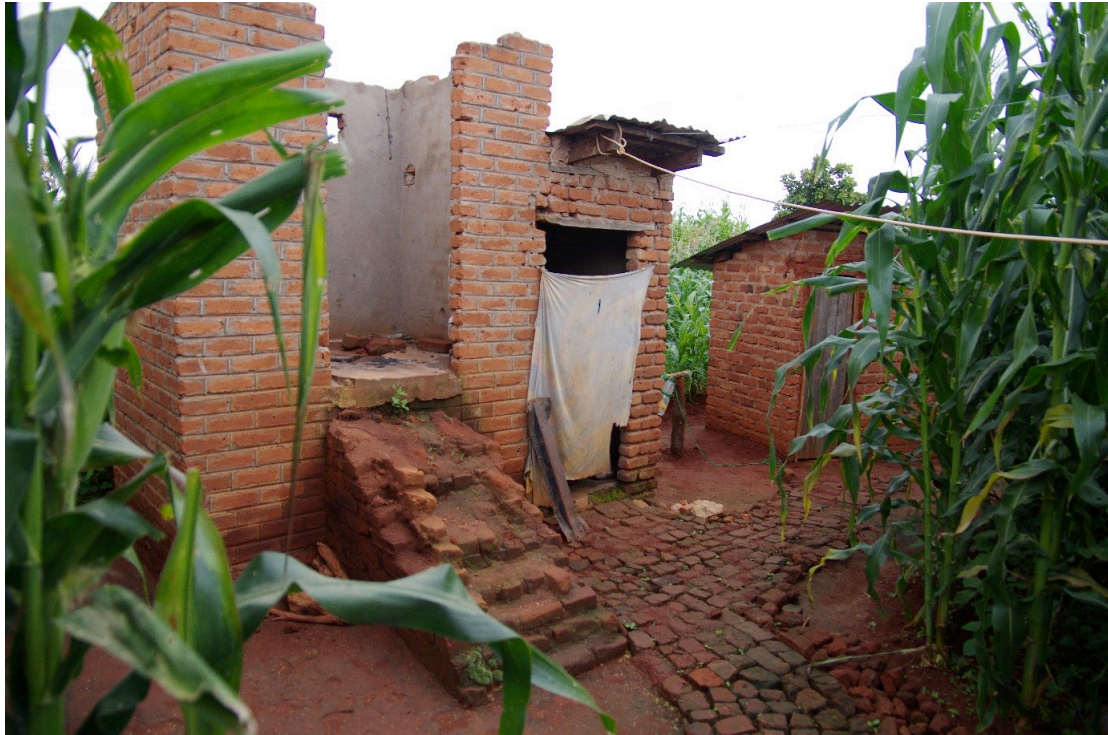
Photograph 1. Abandoned Skyloo and latrine used instead (right)
