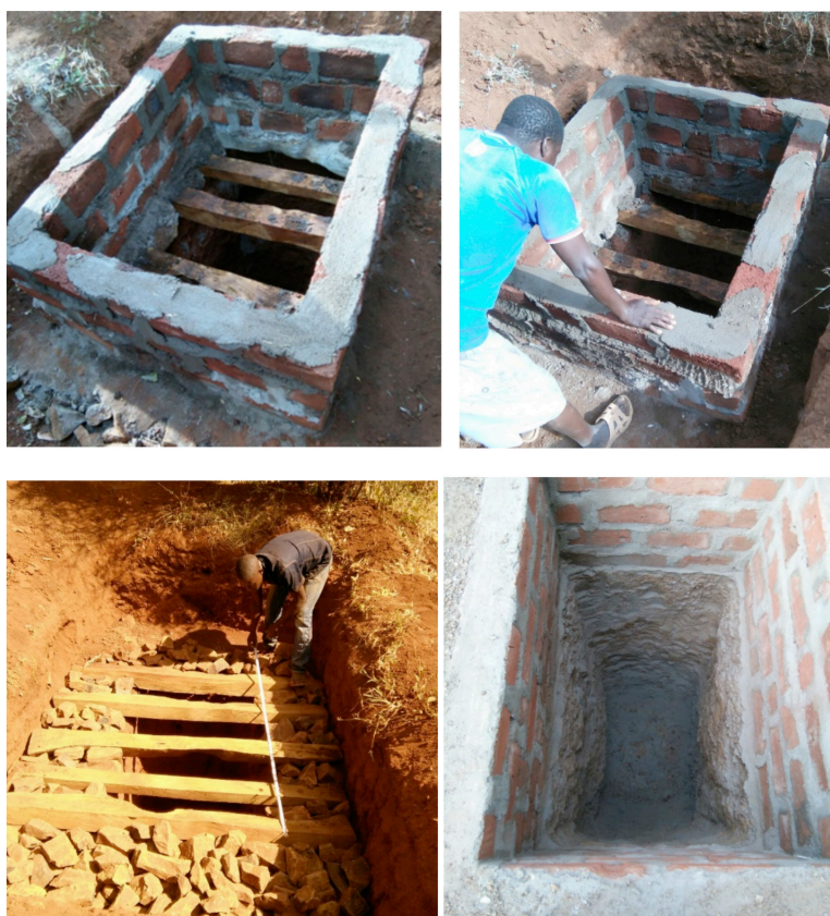
Photograph 1. Images of locally reinforced latrines that ensures stability and sustainability of the latrines
