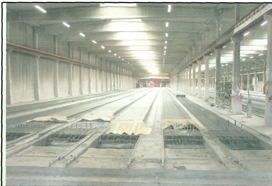
Figure 4.4 Casting beds in a hollowcore production shed (Courtesy of BPCF, 2003)
