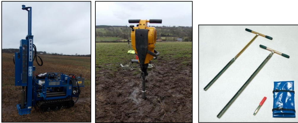
Figure 3.15: The Honda drilling rig at the Arable Site, the Atlas Copco Cobra at the Cattle Site, and a Gouge Auger used at the Horse Site. (Eijkelkamp Agrisearch Equipment, 1999).
