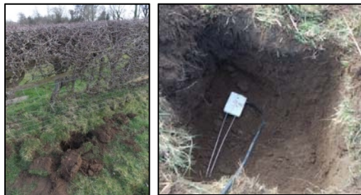
Figure 5.25: Campbell Scientific 616 TDR probes installed at site.
