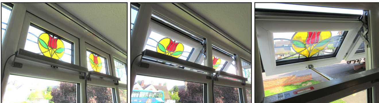
Figure 9. Windows controlled by chain actuators.
