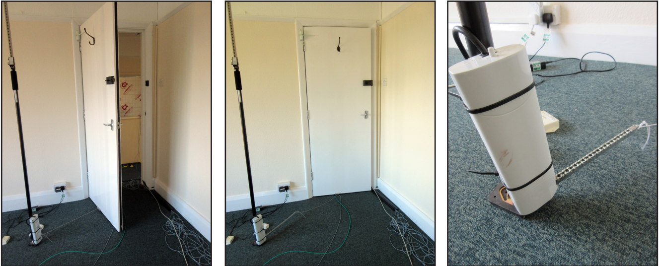
Figure 12. Internal doors controlled by a chain actuator.
