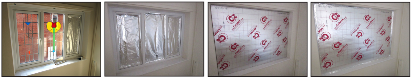
Figure 4. Application of foil and insulation to landing windows to reduce east/west solar gain.
