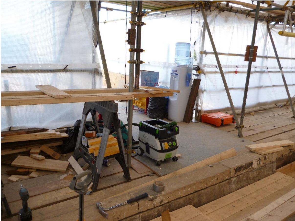
Figure 1 Portable dust extraction is increasingly used in construction to manage dust exposures
