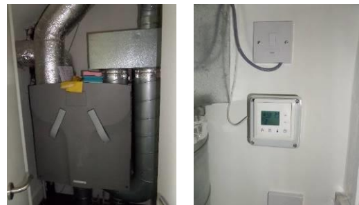
Figure 4-35- MVHR unit located in the cupboard (image on the left) and the control also located in the cupboard (image on the right) (source: author)
