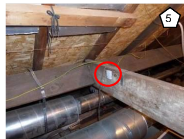
Figure 3-66- Temperature & RH data logger located in the door attic space housing the MVHR unit (part of the thermal envelope) (source: author)
