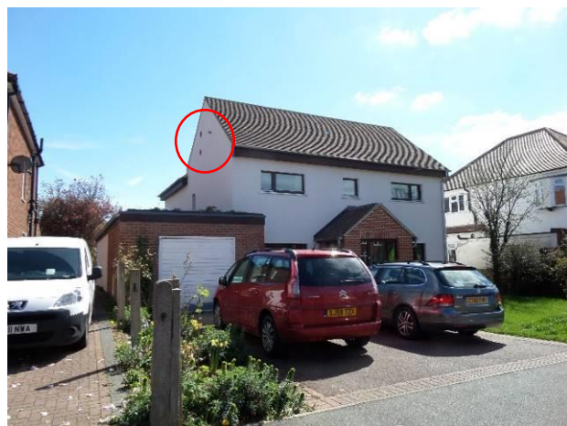
Figure 4-44- View of the building showing the as built location of supply and extract air as well as the boiler flue (source: author)
