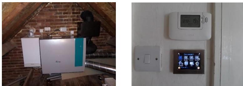
Figure 4-40- MVHR unit located in the loft (part of the thermal envelope) (image on the left) - MVHR control located in the second floor landing (image on the right) (source: author)
