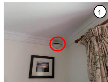
Figure 3-56- Temperature data logger located in the fresh air outlet in the living room (source: author)
