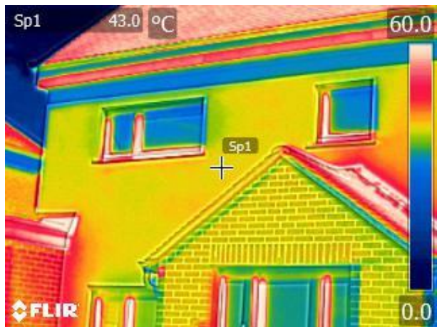
Figure 4-61- Surface temperature reaching 43.0°C measured at 5:00pm (Southwest elevation)
