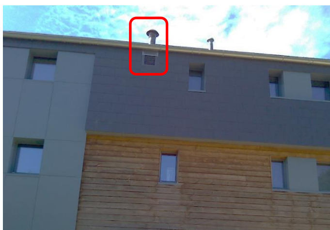
Figure 4-49- Northeast façade indicating the position of the MVHR extract and intake, extract is located on the roof and the intake on the wall below the extract.
