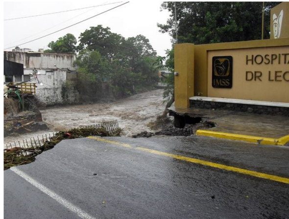
Figure 3: Damage caused to Los Maestros Avenue bridge and Dr. Leonel Ramirez general hospital during Hurricane Jova by the overflow of the Colima river. (Source: El Universal newspaper, October 13, 2011)
