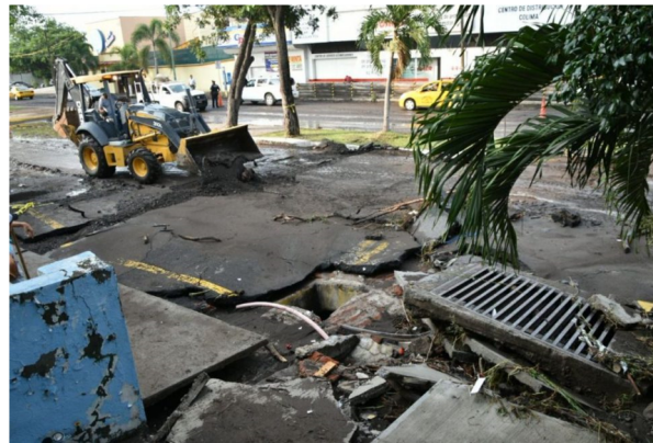
Figure 4: Damage caused to 20 de noviembre Avenue by the overflow of the Manrique brook. (Source: El Diario de Colima newspaper, August 3, 2018)
