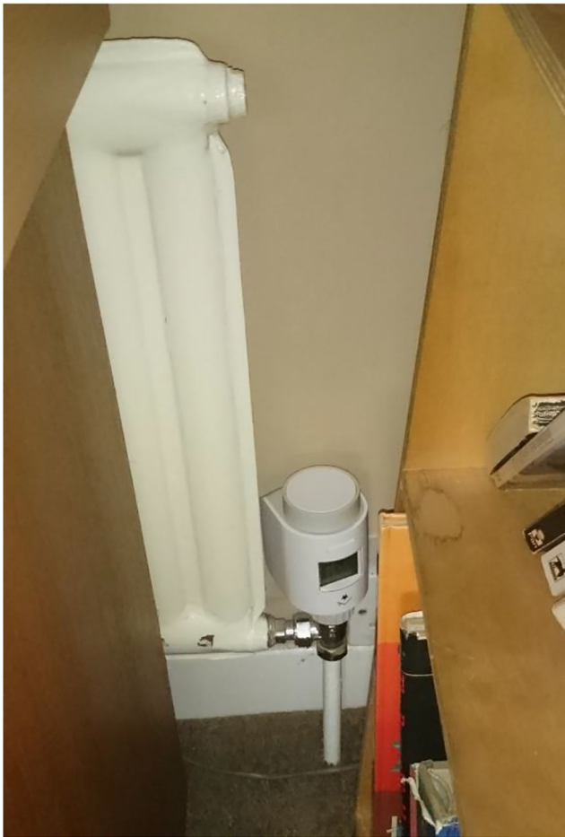
Fig. 1 Providing access to inaccessible controls
