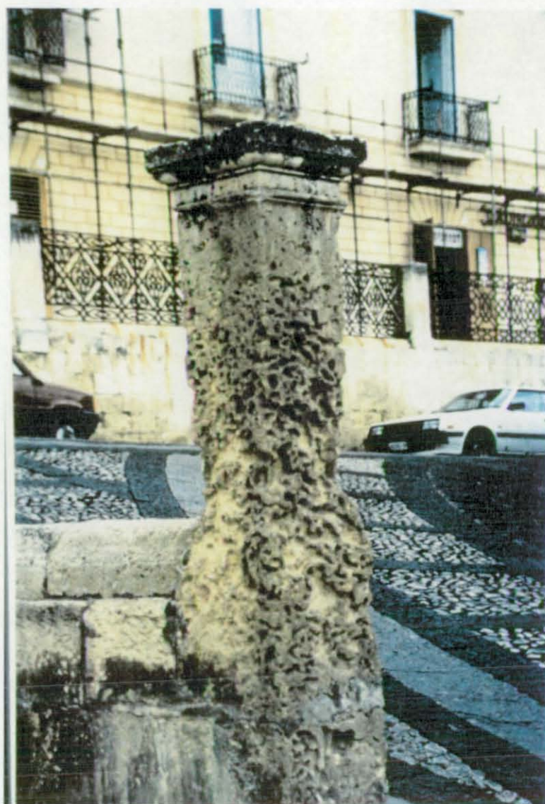
Figure 6.2. Effects caused by alveolation decay on a pillar.
