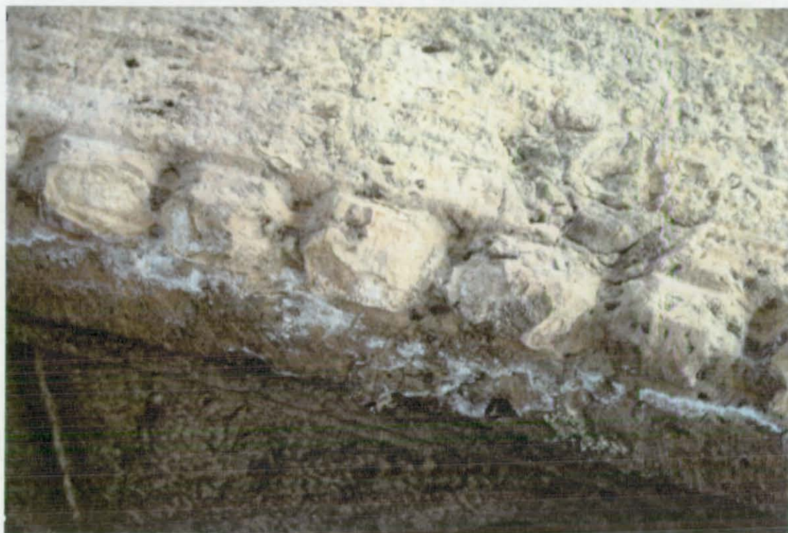
Figure 6.4. Salt efflorescence on a building element made of Angera stone at the "Cortile Richiniano della Ca' Granda" in Milan.
