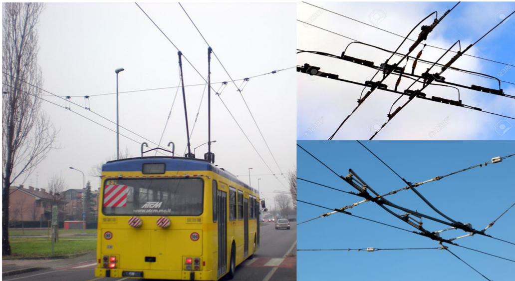
Figure 4.4.5-Three main elements of pure catenary (left) [137], crossing (upper right) [138] and switch (lower right) [139] form trolleybus' catenary system
