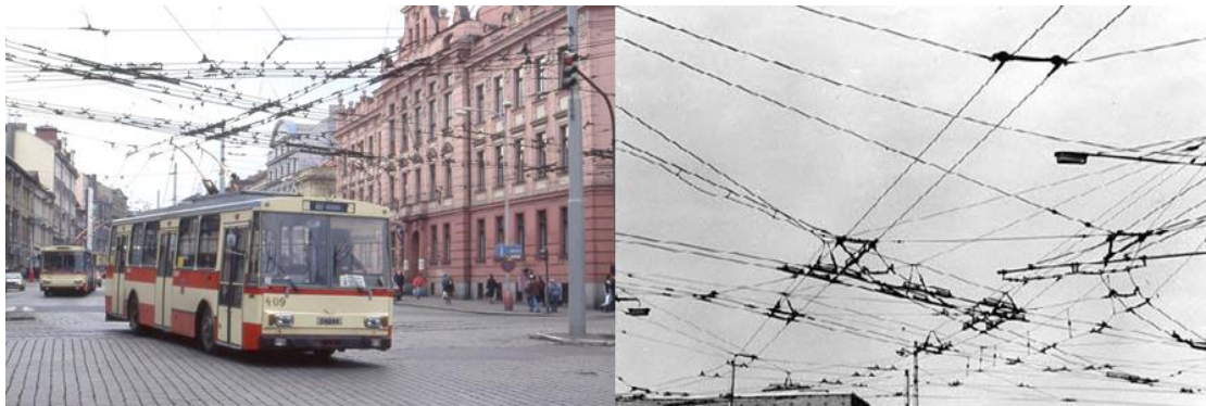
Figure 1.2.5 Complicated trolleybus overhead line webs at crossroads [16] [17]
