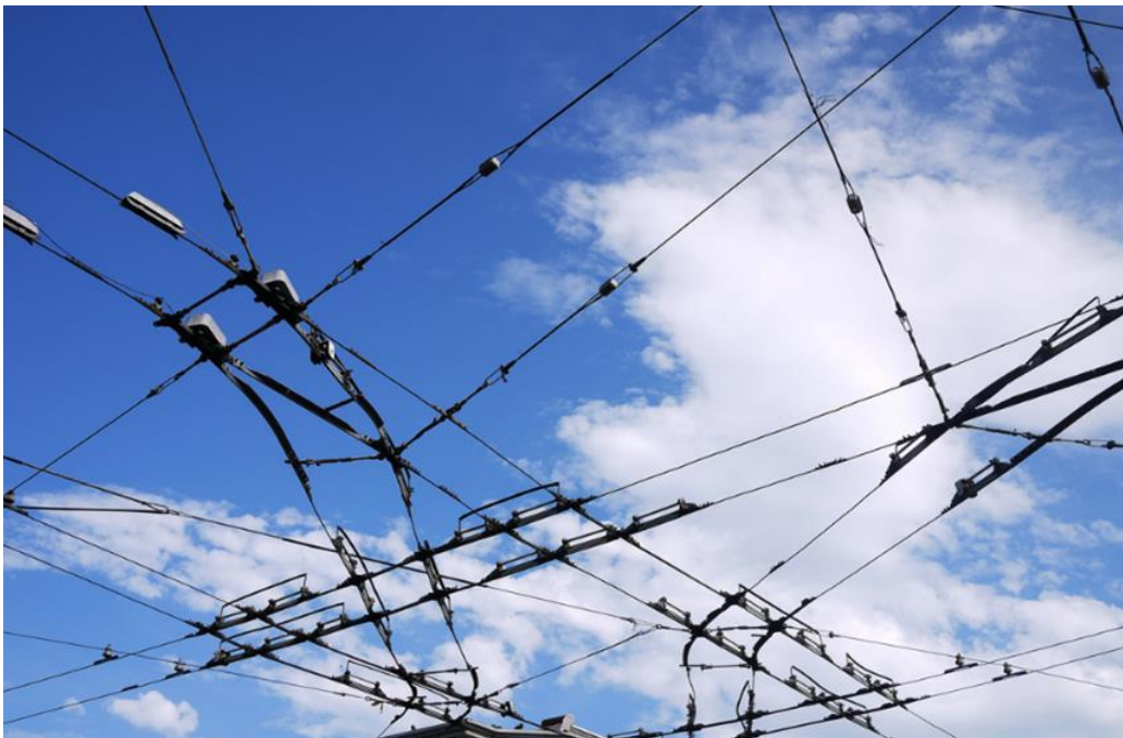
Figure 4.4.6-Complex catenary at crossroad [140]
