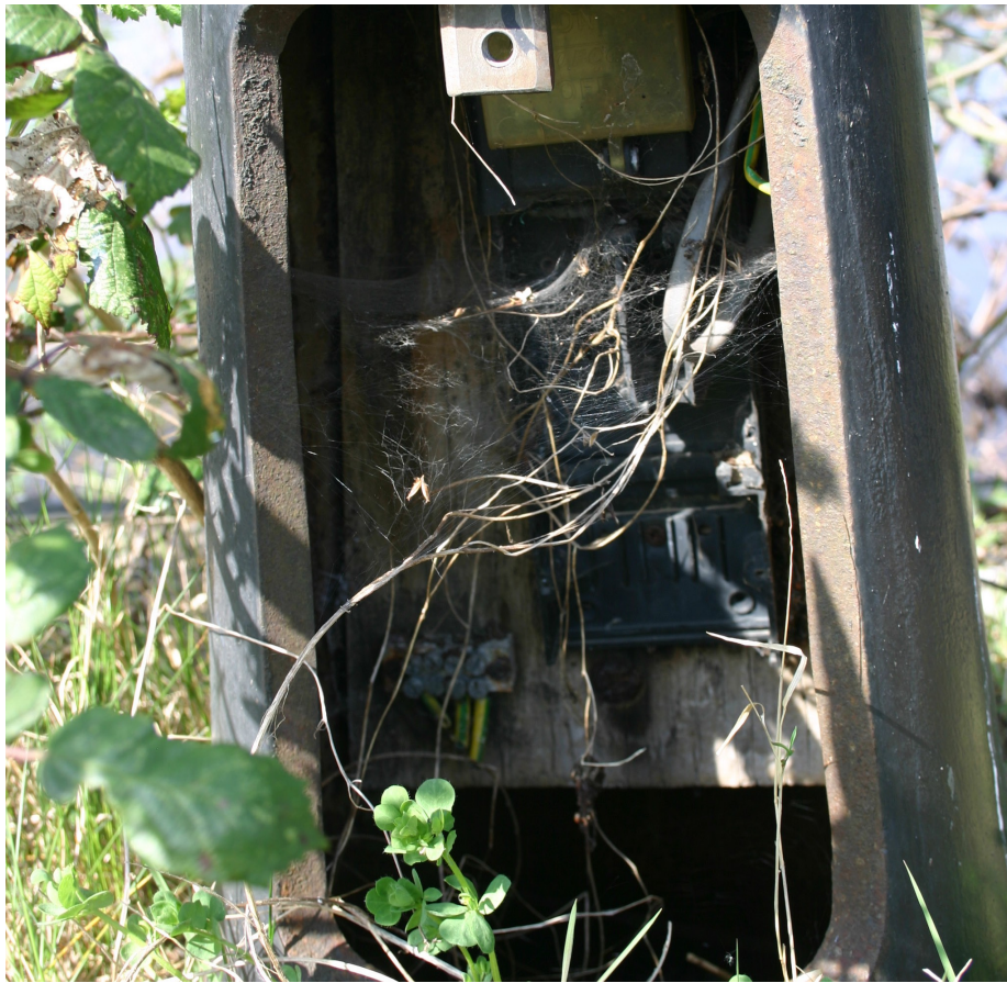
Figure 3. Web/sites. Plants, spiders and electric wiring in an old lamppost on the promenade of Pomona Strand. 4th April, 2019.
