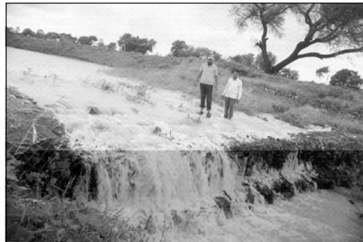
Overflow from Gabion outlet
