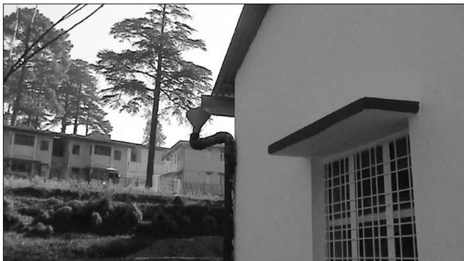
Figure 7. Rooftop rainwater harvesting at VPKAS, Almora
