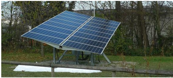
Figure 1a: The tracker PV-installation with 4,8 kWp serves as a tracker reference station on the BFH Campus.
