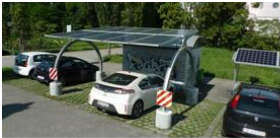
Figure 1b: The new solar carport-installation with 2,9 kWp was installed in 2013 on the BFH Campus and serves as a test station for new equipment.
