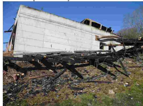
Figure 10: Workshop after the fire seen from east (position of the photographer first red circle on the map)
