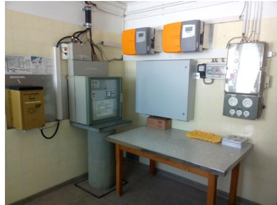
Figure 3: Grid-connection of new PV modules mounted at Jungfrauoch in 2014 (right), next to old ASP inverter from 1993 (left).
