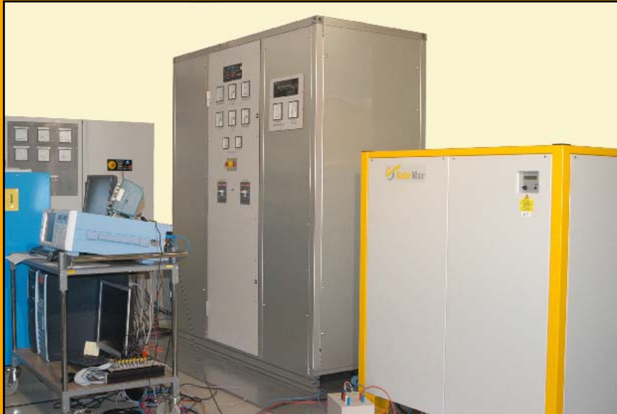
BFH-TI's 100 kW PV array simulator shortly before it became operational in 2009
