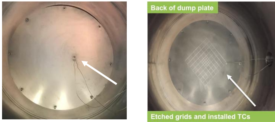
Figure 3.3. Non-plasma facing sides of the currently installed (left) and previously installed (right) dump plates. White arrows point out installed thermocouple locations. Etched gridlines visible on old dump plate.
