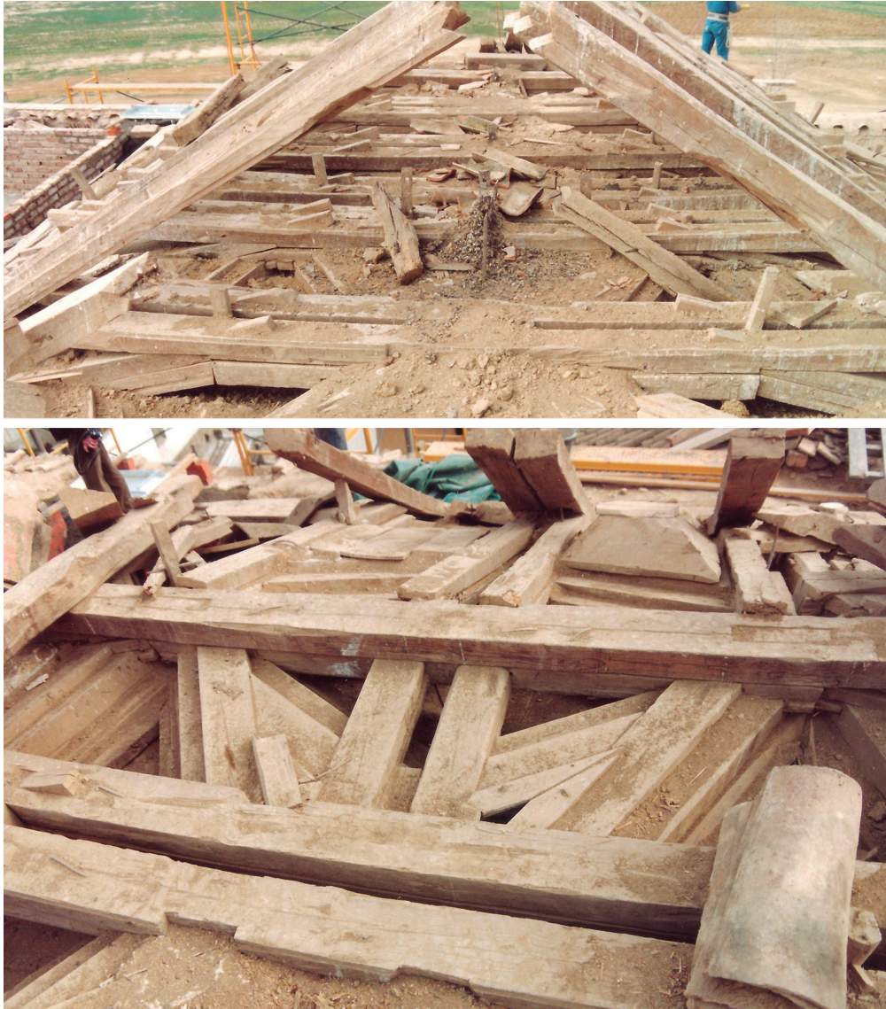
Figure 7. Details of the original structure in its state during the 1991 restoration works. Above: rafter pitches with higher ends birdsmouth cut to accommodate a lost ridge beam. Collar beams and under-rafters can also be observed. Below: Short side of the rectangle from the top plane or almizate . The picture shows the short struts between under-rafters forming 4 point stars on the top plane. On the descending panel, a rhombus based coffer can be seen upon the struts between under-rafters. The rafters upon these, perpendicular to the main ones, are cut a little above the joint.
