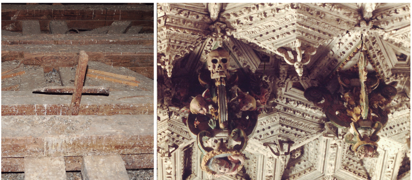
Figure 10. Left: View of the wooden bars used to hang the convex coffers and pendants. Right: Fleurons, carvings and three large pendants hanging from the top horizontal plane.
