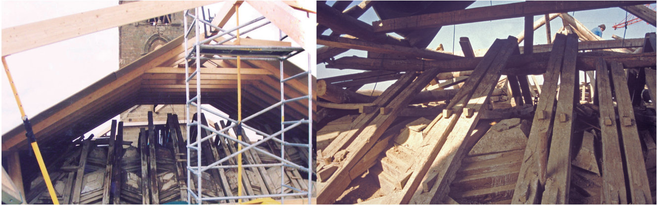
Figure 2. Exterior view of the ceiling during the 1991 restoration works directed by architect M.C. Fernández-Cabo and carried out by builder J. Alonso, REARASA Company.
