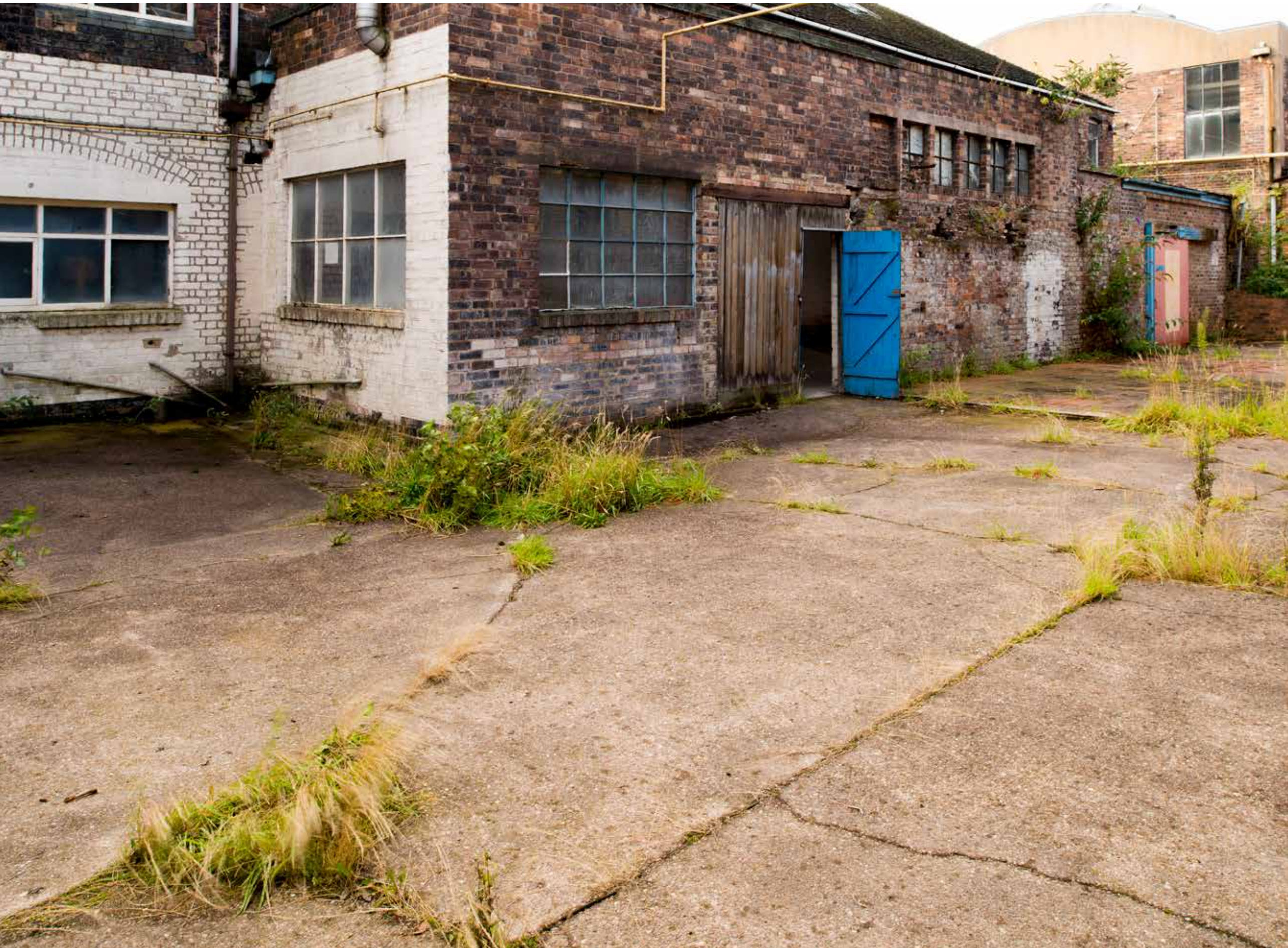
Fig. 4. Former Spode Works where concrete foundations show the trace outline of a bottle kiln and other earlier structures
