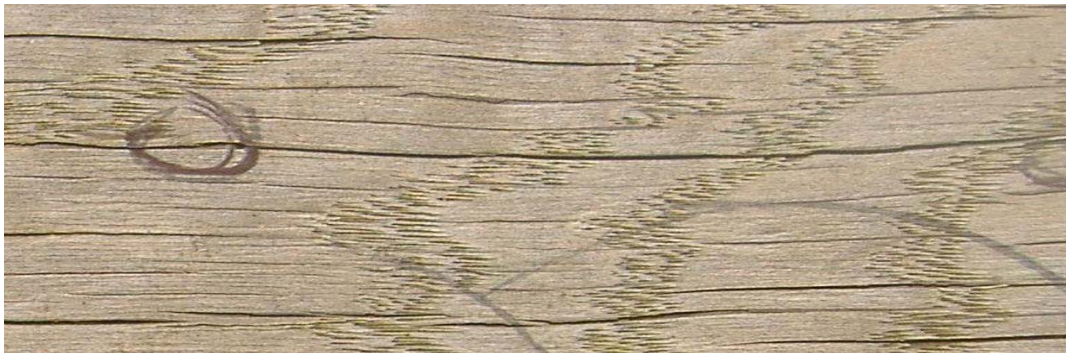
Figure 4.48 Checking on the surface of an untreated oak cross-piece in December 2006.
