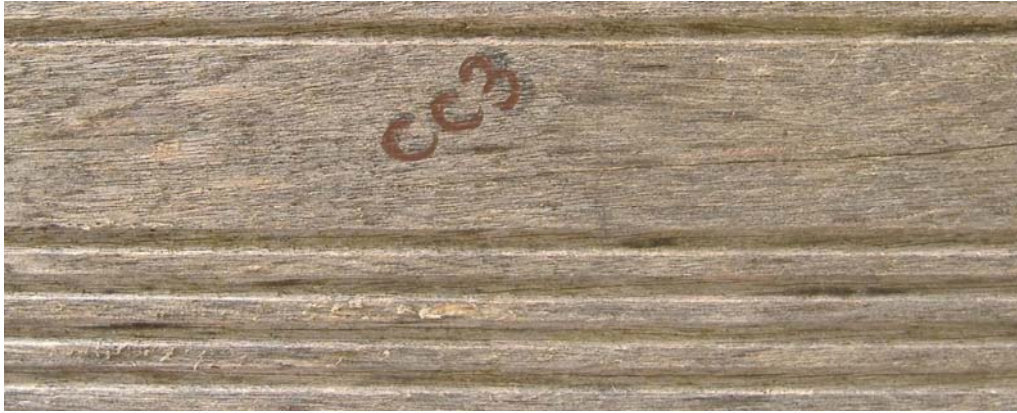
Figure 4.49 Stain on the surface of an untreated esa decking board.
