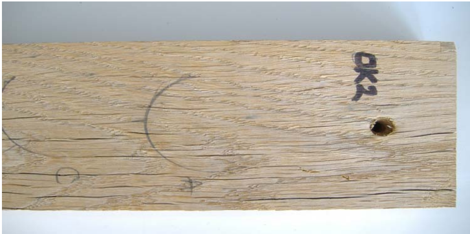
Figure 4.47 Checking on the surface of an untreated oak cross-piece in September 2006.
