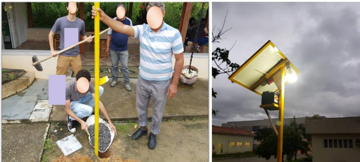
Figure 2. Images of the solar panel project in its final assembly. Some parts of the images were covered to protect identities and advertisements
