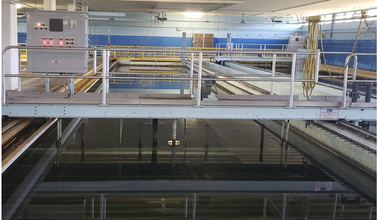
[ Insert Figure 45. Rectangular Automatic Backwash Filter Installed at Lowell Regional Utility, Massachusetts, USA for Dual Media Filtration (Credit: Superintendent Steve Duchesnel, LRU, August 2019) (236) ]
