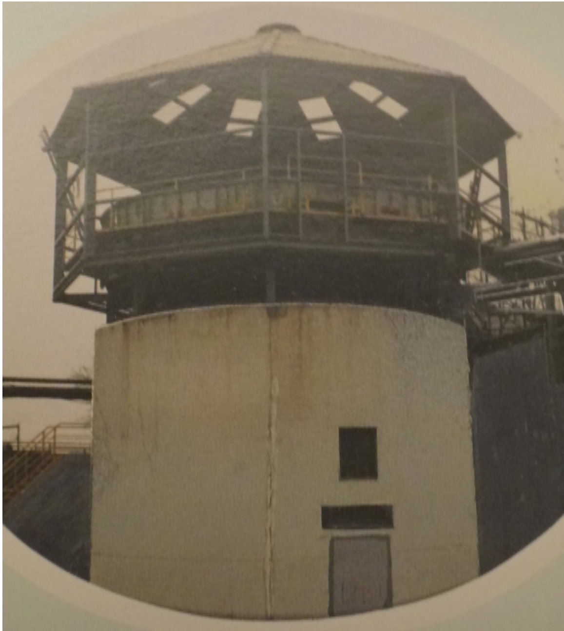
[ Insert Figure 34. Construction of a 30-ft diameter DAF-filtration (DAFF; Sandfloat) unit on the top of an existing sedimentation clarifier in Berlin, Germany ]
