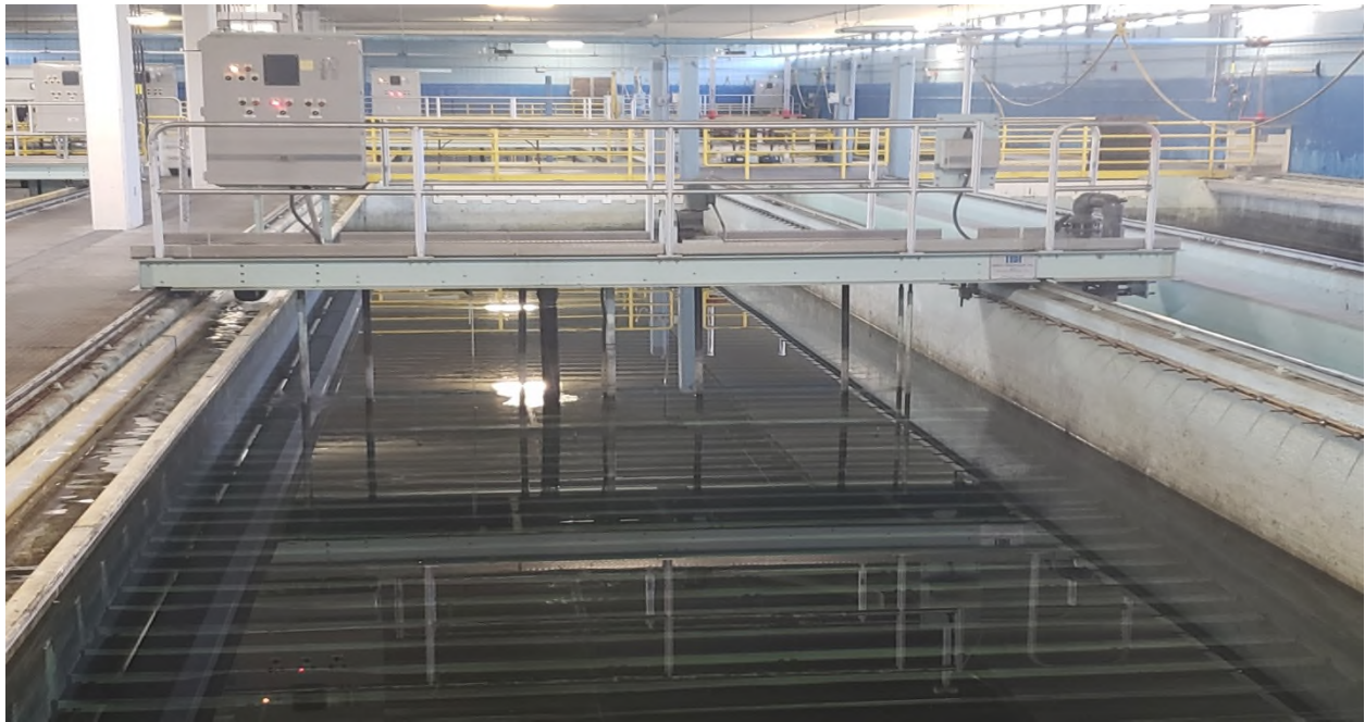
[ Insert Figure 46. Rectangular Automatic Backwash Filter Installed at Lowell Regional Utility, Massachusetts, USA for Granular Activated Carbon Filtration (Credit: Superintendent Steve Duchesnel, LRU, August 2019) (236) ]
