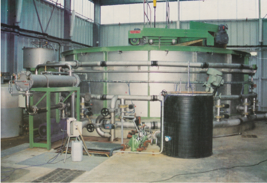
Figure 2. A full-scale DAF-filtration water treatment plant (Krofta Sandfloat Type SAF-BP-24; 24-inches diameter)
