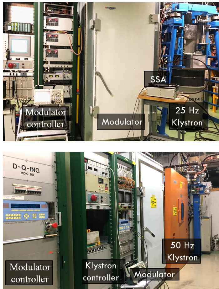
Figure 2.6: Picture of the HPRF of the S-band test stand before (top) and after (bottom) upgrade: klystron, modulator and control system.
