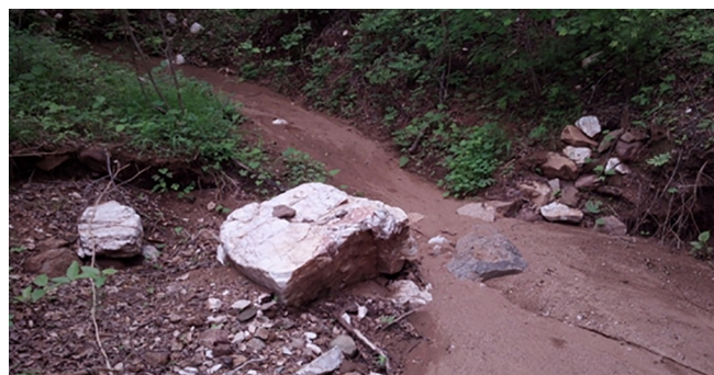
Fig. 3. Stone check dam failure (broken) in the Culiacán watershed (Mexico).
